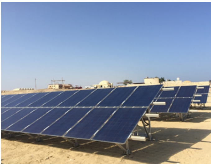
Fig. 2: Solar panels at Oasis Hotel
