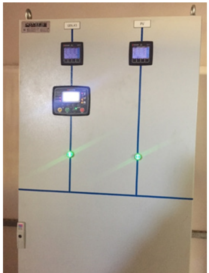
Fig. 5: Controller at Oasis Hotel
