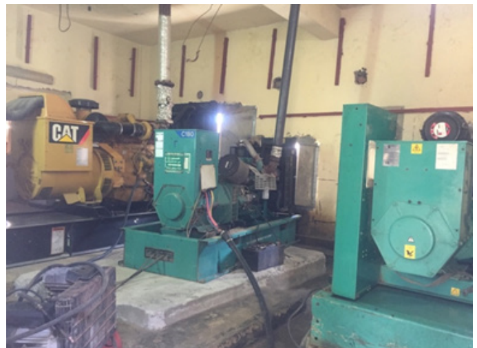
Fig. 3: Diesel generators at Oasis Hotel
