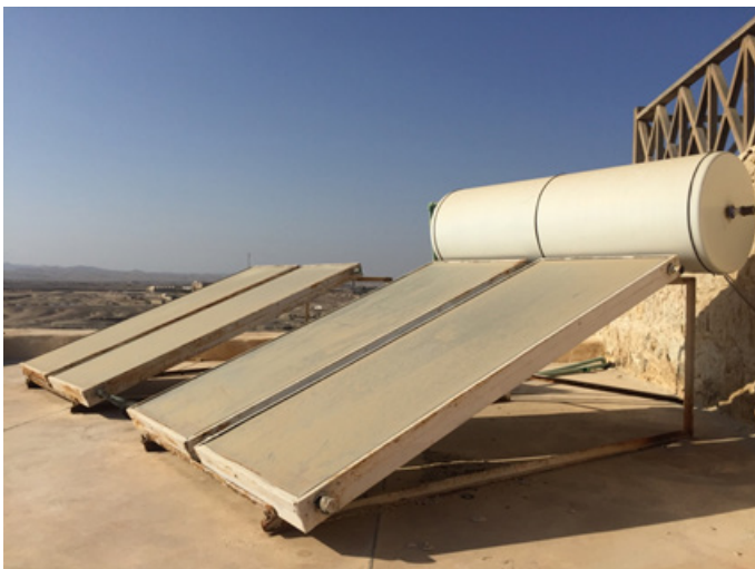
Fig. 4: Solar water heaters at Oasis Hotel
